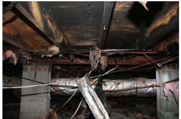
Figure 1: Crawl Space Fire Example
