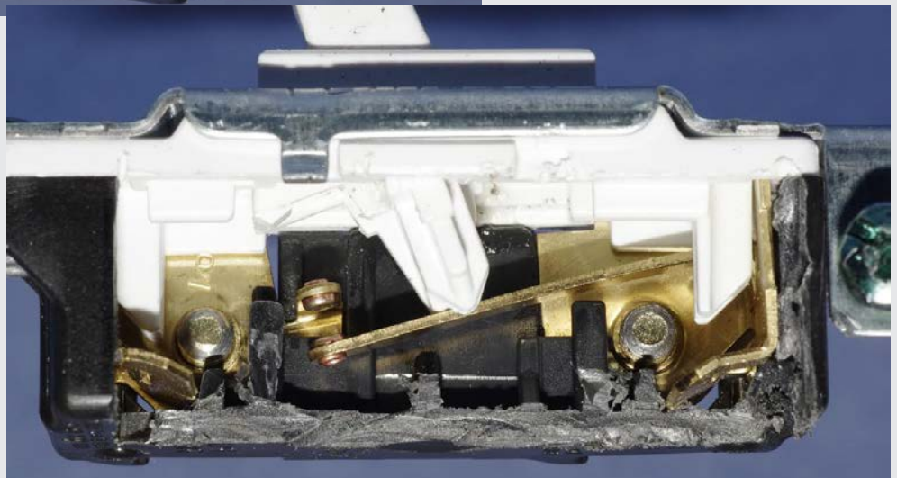
Typical Single Pole Residential Switch in the OFF Position
